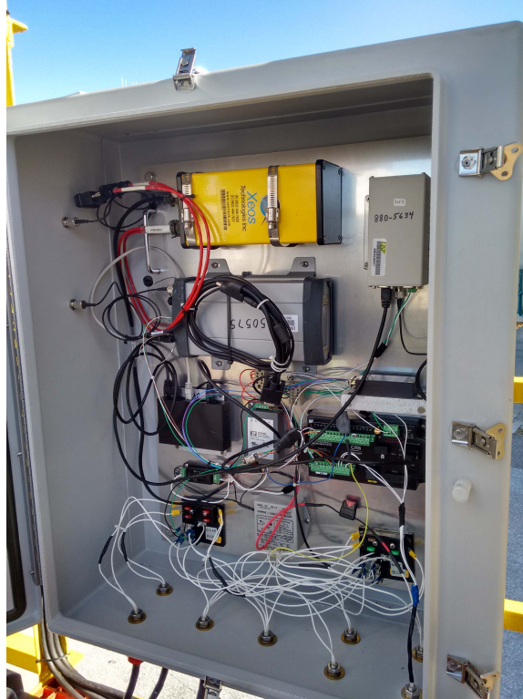
Figure 4. GPS and related electronics in the weather-proof enclosure, mounted on the buoy superstructure.
